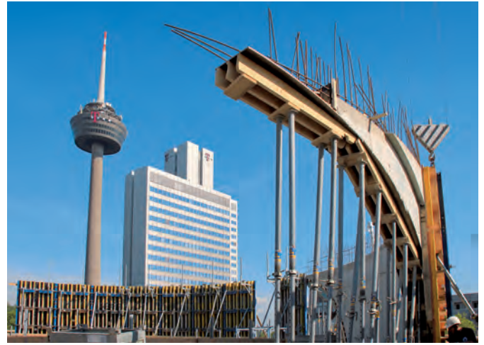
Fig. 3. An experienced supervisor supports site staff when handling formwork for such non-standard component geometries (photos: Doka)
