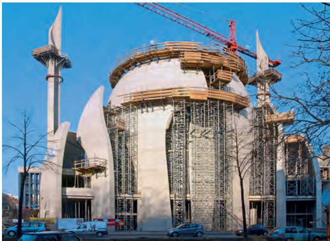
Fig. 2. More than 2000 m 2 of special formwork in single and double curvature pre-assembled with millimetre accuracy by the Doka “ready-to-use” service for the complex dome geometry
