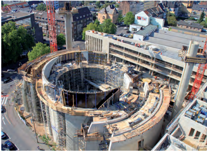
Fig. 1. The mosque challenge: several concrete shell segments gradually growing together as they rise to form the central dome
