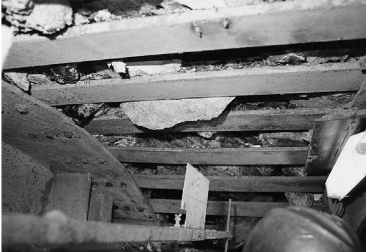
Figure 10-2 Trailing fingers of a gripper TBM ( \varnothing 5.2 m) in a fractured phyllitic Verrucano, Illanz II
