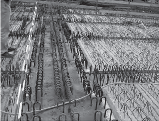
Figure 4.3 Precast concrete floor plates with in situ concrete topping supported on primary and secondary downstand beams.
